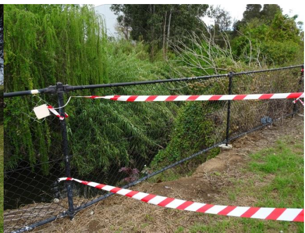
Erosion between sportsground and creek bank
