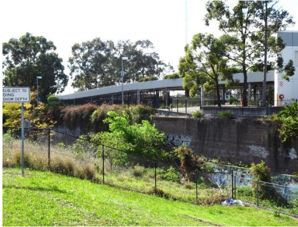
Channelised creek is subject to flooding
