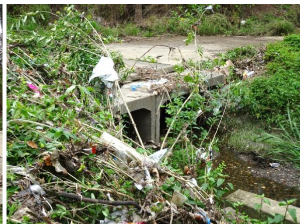
Rubbish at causeway after rain
