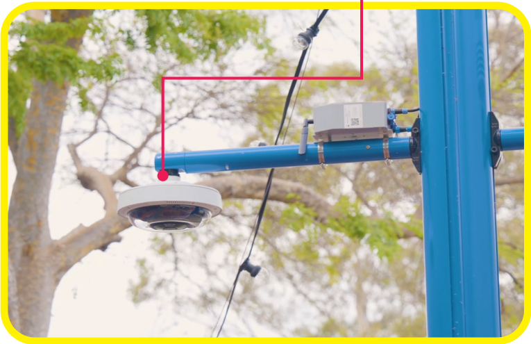
CCTV Camera Type
