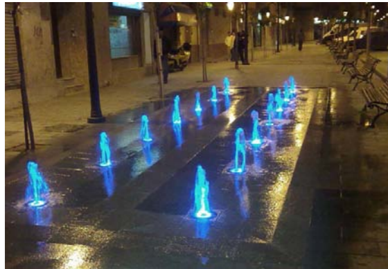
ZERO DEPTH WATER PLAY FEATURE (feature lit at night)
